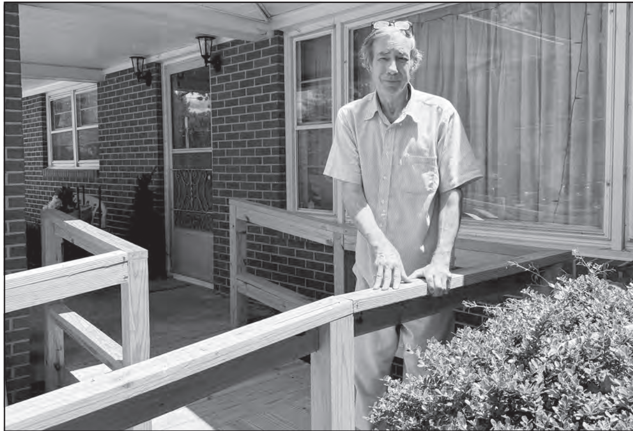
This wheelchair ramp, constructed by volunteers from United Methodist Church in Archdale, has improved Dan's quality of life and greatly increased his safety and independence. Dan enjoys people and this ramp allows him more opportunities to attend church, get fresh air, and engage with his community.
